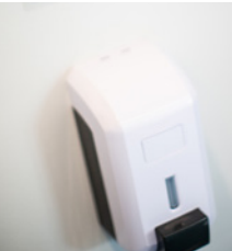
Installation of hydroalcoholic gel throughout the facilities
